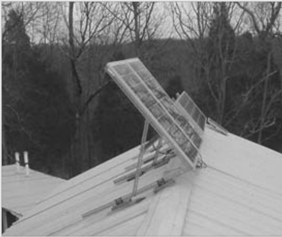
Figure 12.17: PV panels power the Schimmoeller-Lindbergh residence, Andy McDonald
