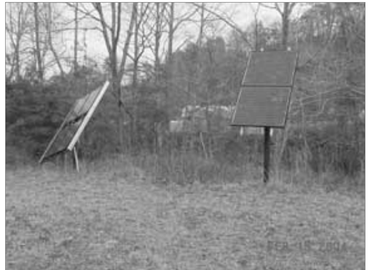
Figure 5.3: The tracking PV array on the left is facing the afternoon sun, while the fixed array on the right faces due south, Andy McDonald
