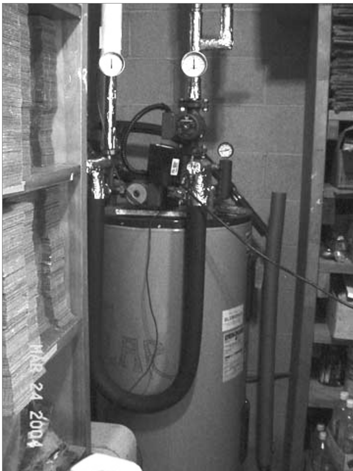
Figure 7.6: A conventional electric water heater tank uses an external heat exchanger in the solar water heating system at the ASPI office in Mt. Vernon, Kentucky, Andy McDonald
